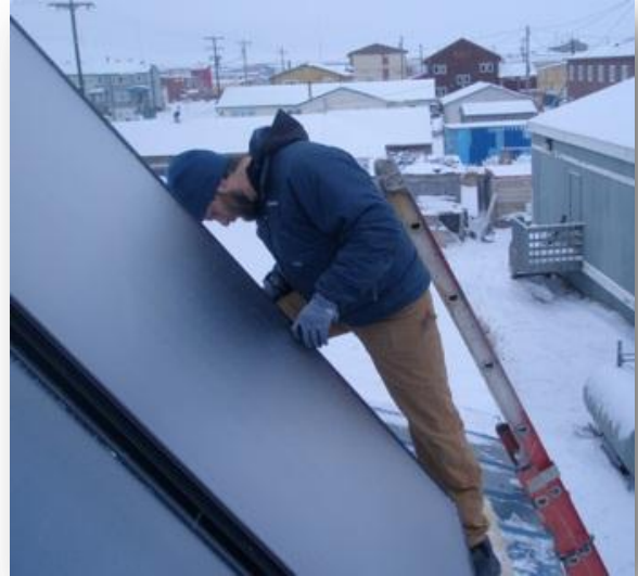
Jesse Logan (KEA) adjusts a flat plate solar thermal panel on Mary Omnik's house. Photo courtesy of KEA.
